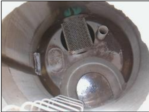
Figure 6.9: A view of an Oil Grit Separator from a maintenance manhole.
