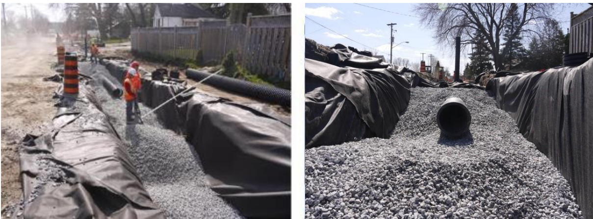
Figure 6.7: Perforated Pipe installed adjacent to the roadway as part of a bioswale design
