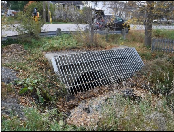
Figure 6.48: Storm sewer inlet at Mildred St.
