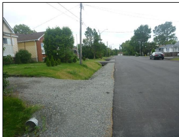
Figure 6.30: Example of a rural cross section (ditches) along Roger Street in Sudbury
