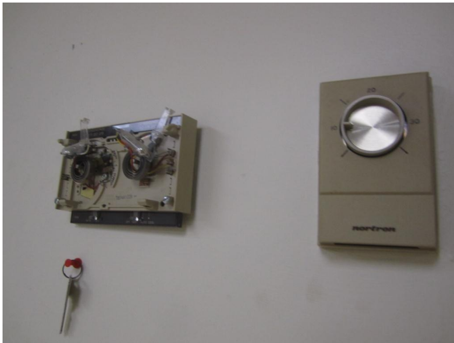
Photograph No. 4. Typical mercury containing thermostat found throughout building.
