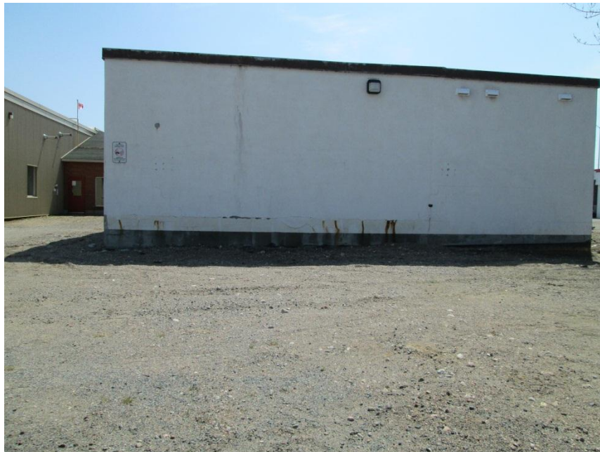
Photograph No. 2. Asbestos containing “stucco” parging in poor condition, along exterior of Site building.
