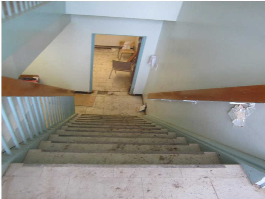
Photograph No. 6. Lead containing light green and dark green paint found throughout building.
