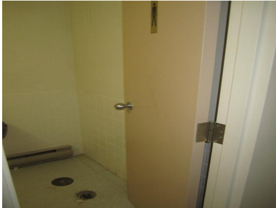
Photograph No. 7. Lead containing light brown paint found on South basement bathroom doors.
