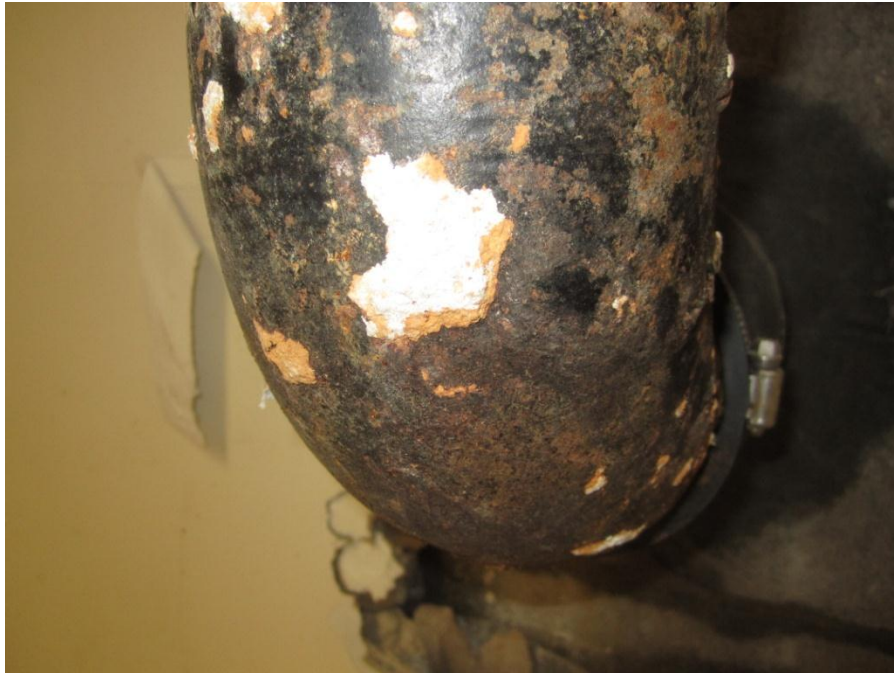
Photograph No. 3. Asbestos containing “plaster elbow” remnants noted in North basement.
