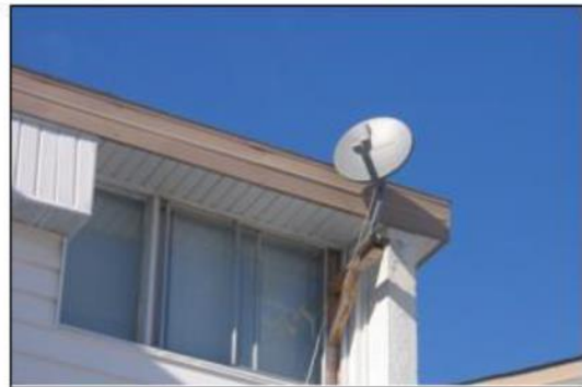
Interferes with Window Operation
