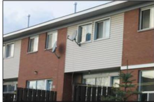
Fastened to Siding
