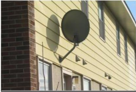
Fastened to Siding
