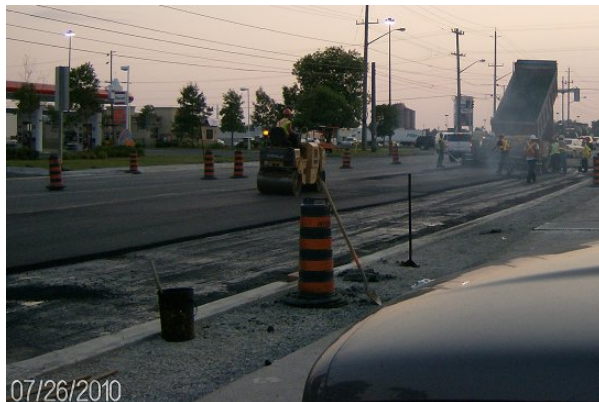
Exhibit 1 – Inferior Asphalt Supplied
