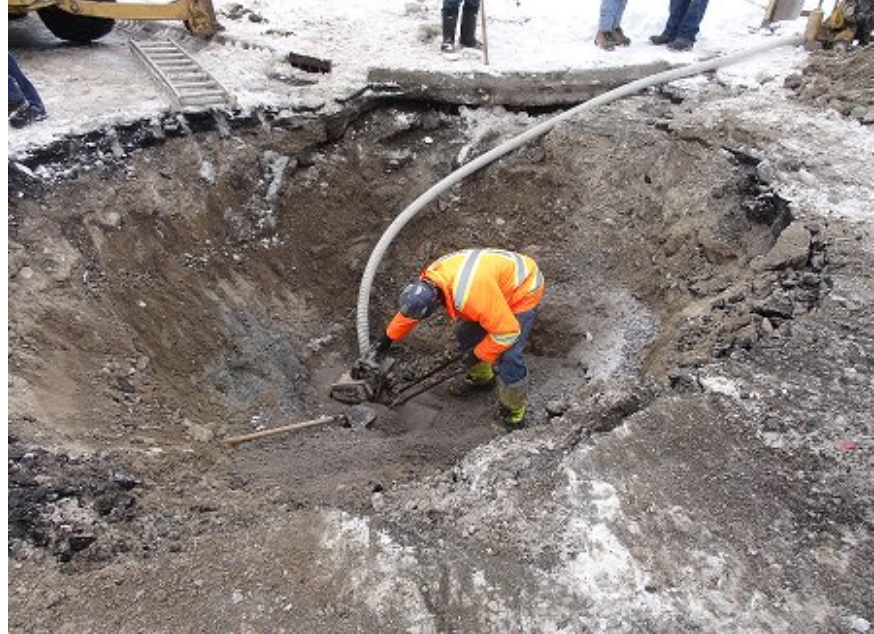
Exhibit 2: Slope Excavation (5 ft depth) in accordance with The Act (Method A or B)
