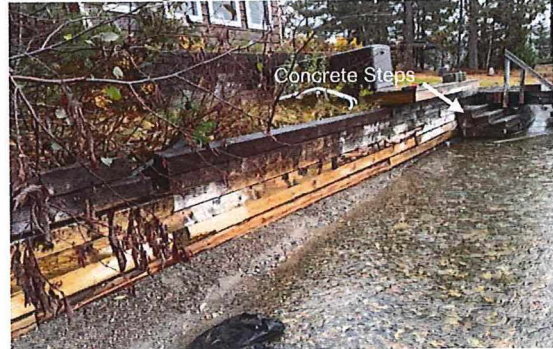
Photo 6. Wall sits on beach and is not counter sunk. Timber somewhat worn by abrasion, but otherwise in good condition.
