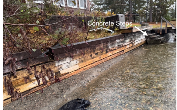
Photo 6. Wall sits on beach and is not counter sunk. Timber somewhat worn by abrasion, but otherwise in good condition.
