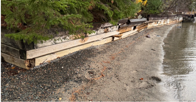
Photo 5. Timber wall with protective beach. Partially collapsed portion of wall near middle.
