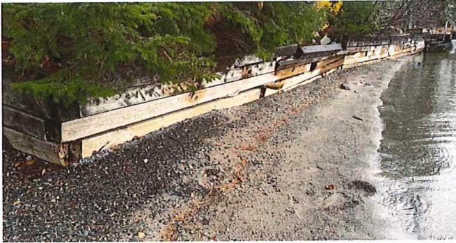
Photo 5. Timber wall with protective beach. Partially collapsed portion of wall near middle.
