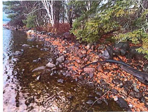
Photo 2. Boulder toe at base of bluff
