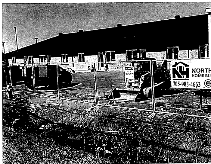
Figure 5 – Row dwelling complex currently under construction directly west of the Subject Lands
