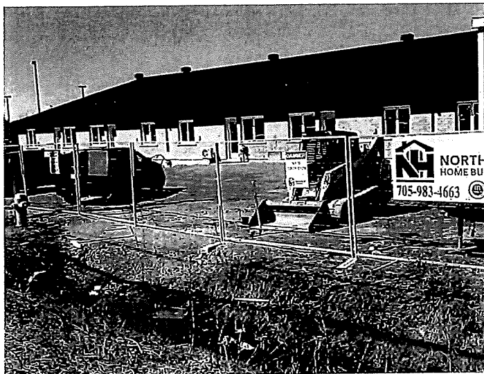
Figure 5 – Row dwelling complex currently under construction directly west of the Subject Lands
