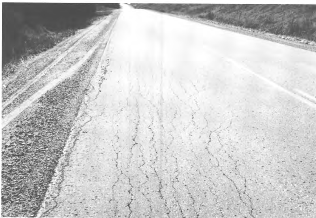
Severe Longitudinal Outer Wheel Track Crack Progresses into Moderate Alligator Crack
