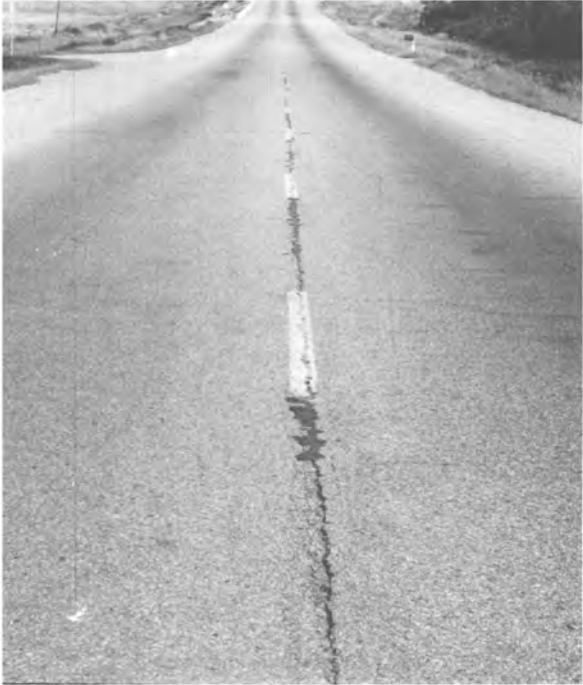
Slight Centre Line Crack
