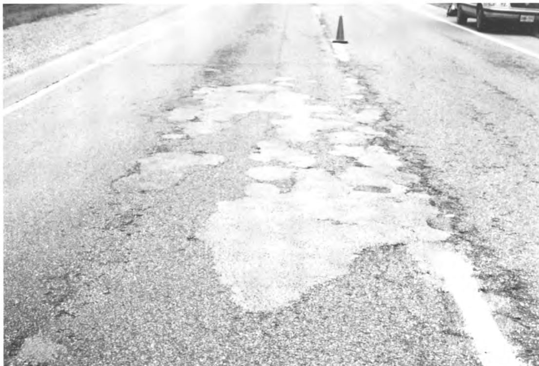
Moderate Distortion from Ravelling and Improper Maintenance Treatment
