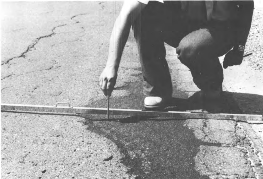
Severe Distortion from Lack of Structural Strength
