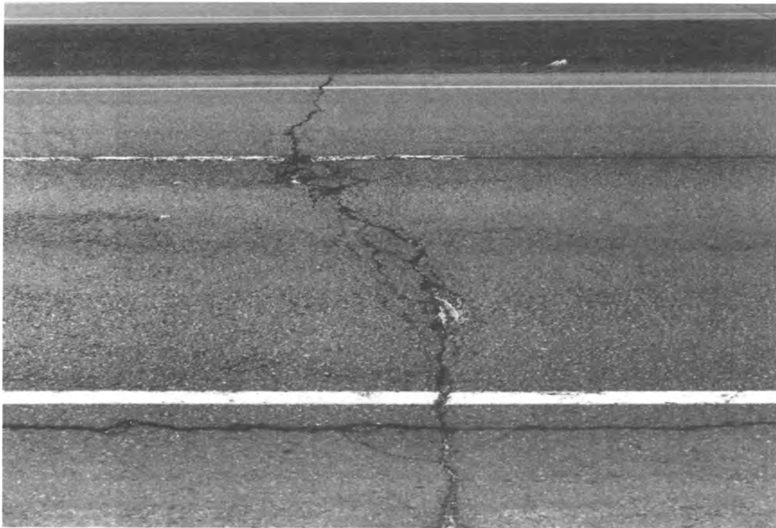
Very Severe (Multiple) Transverse Crack with Spalling
