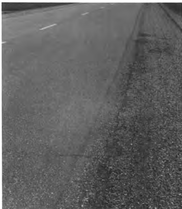
Edge Breakup of Stabilized Shoulder
