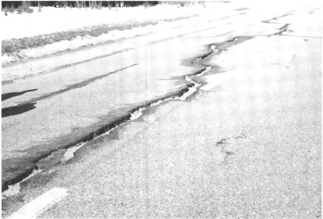
Very Severe Meandering Crack (Single greater than 25 mm)
