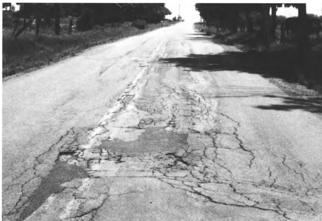
Riding Condition Rating: Very Poor
