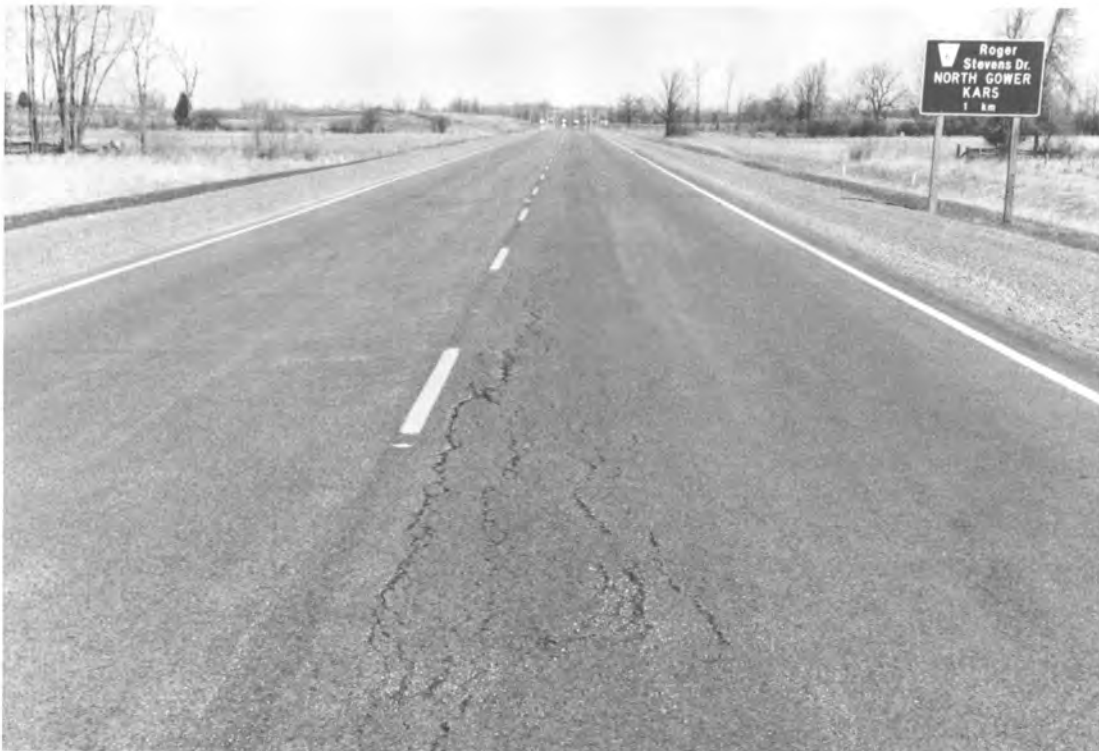
Moderate (Multiple) Longitudinal Wheel Track Crack
