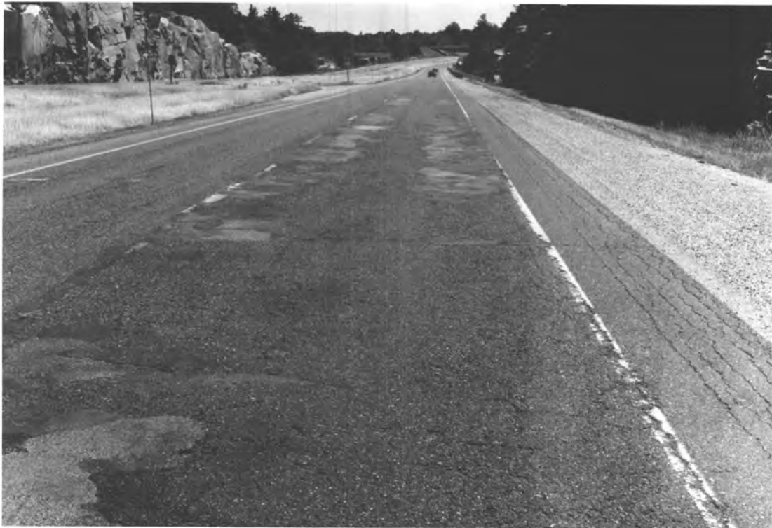
Severe Distortion from Ravelling with Improper Maintenance Treatment
