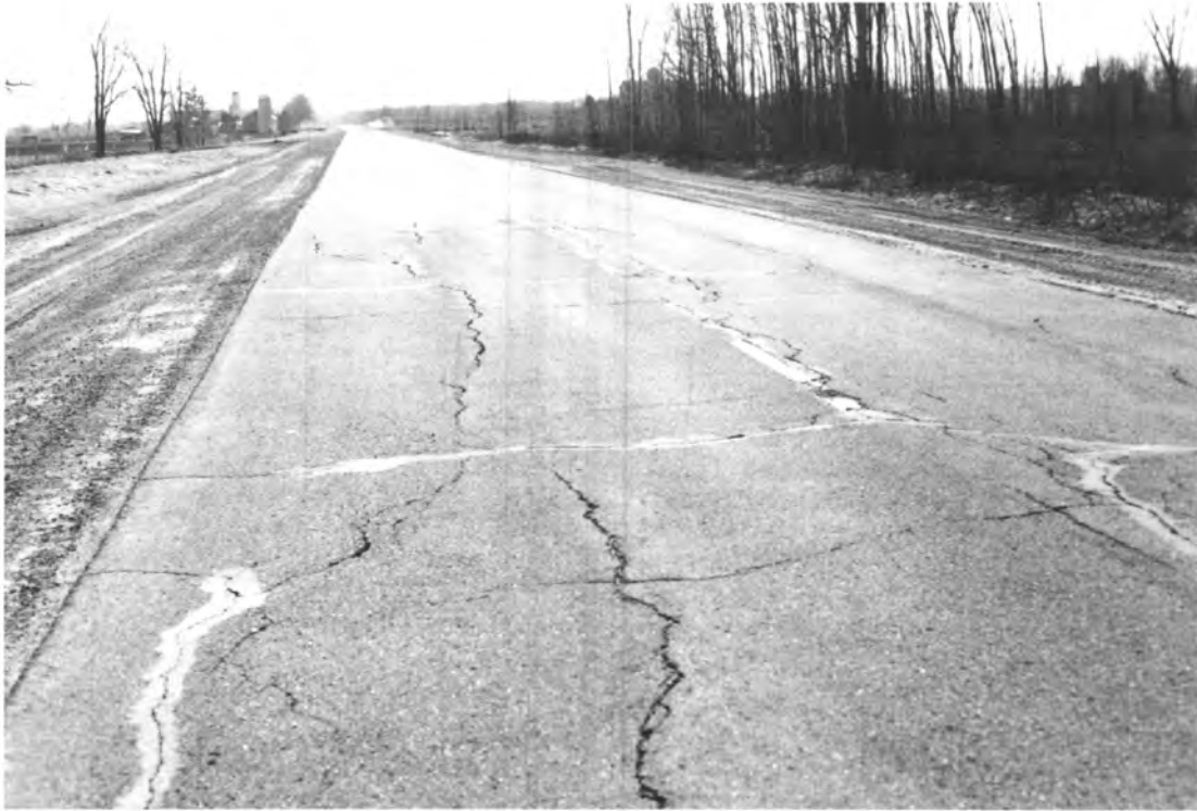
Severe Map Crack
