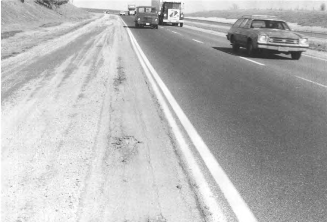
Pavement Edge Paved Shoulder Separation
