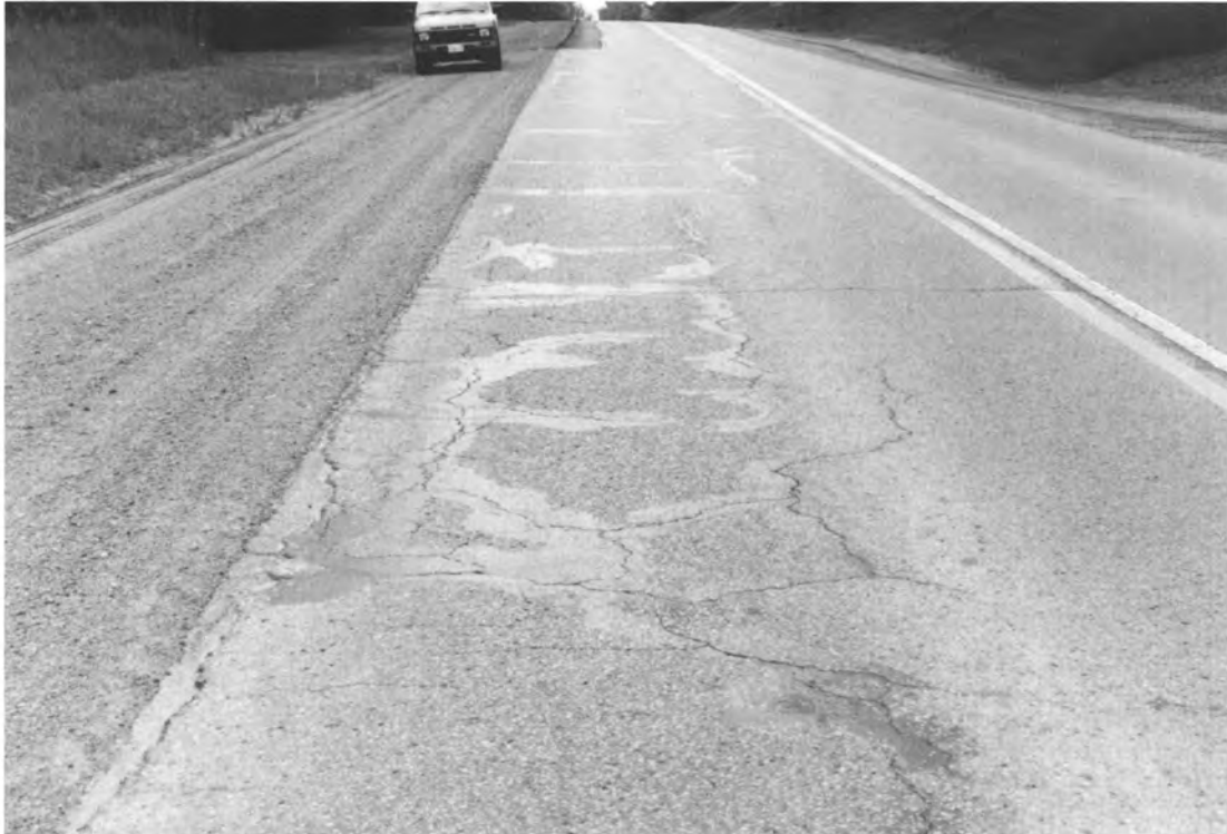
Slight Map Crack
