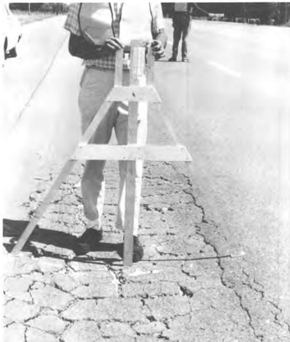
Severe Alligator Crack *
