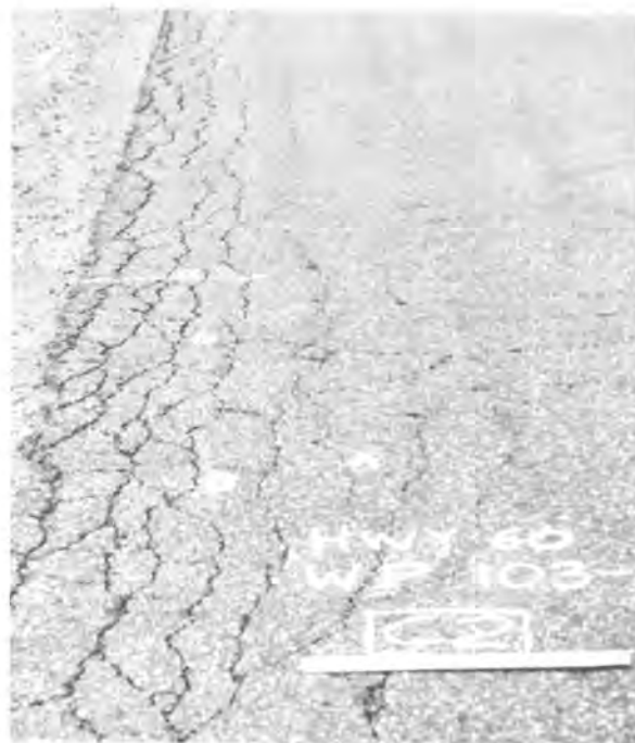
Severe (Multiple) Pavement Edge Crack
