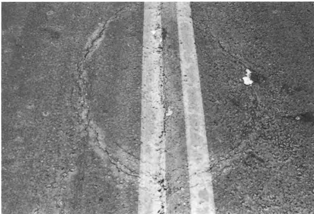
Slight Elephant Footprint Crack
