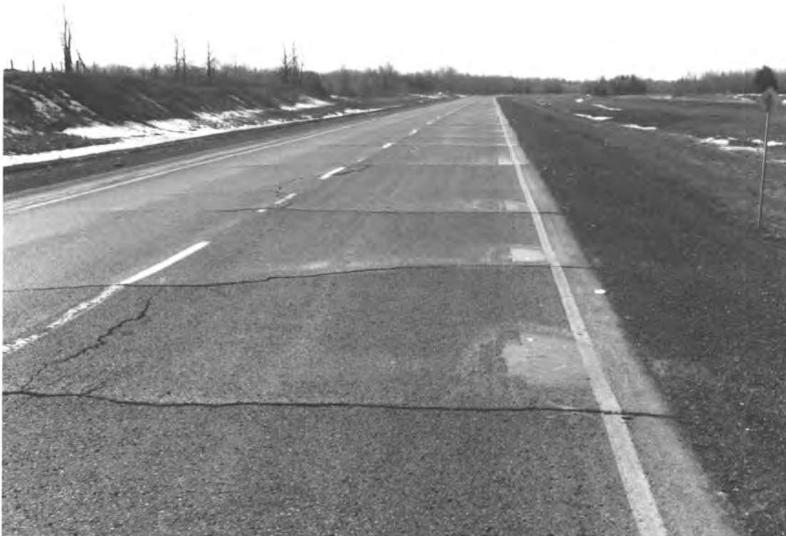
Very Severe Distortion from Transverse Crack Lipping
