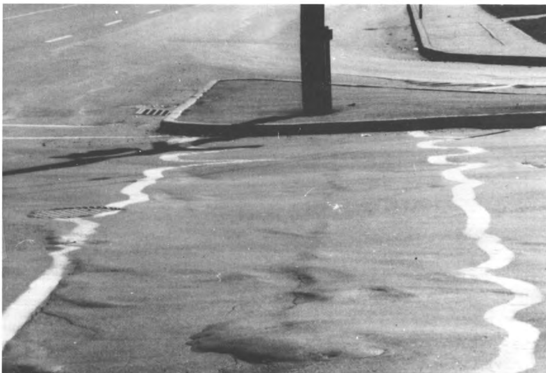
Very Severe Shoving
