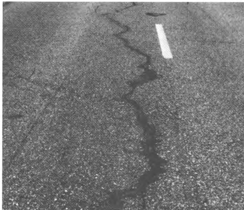
Severe Meandering Crack
