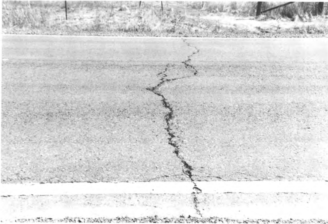
Severe Transverse Crack with Spalling
