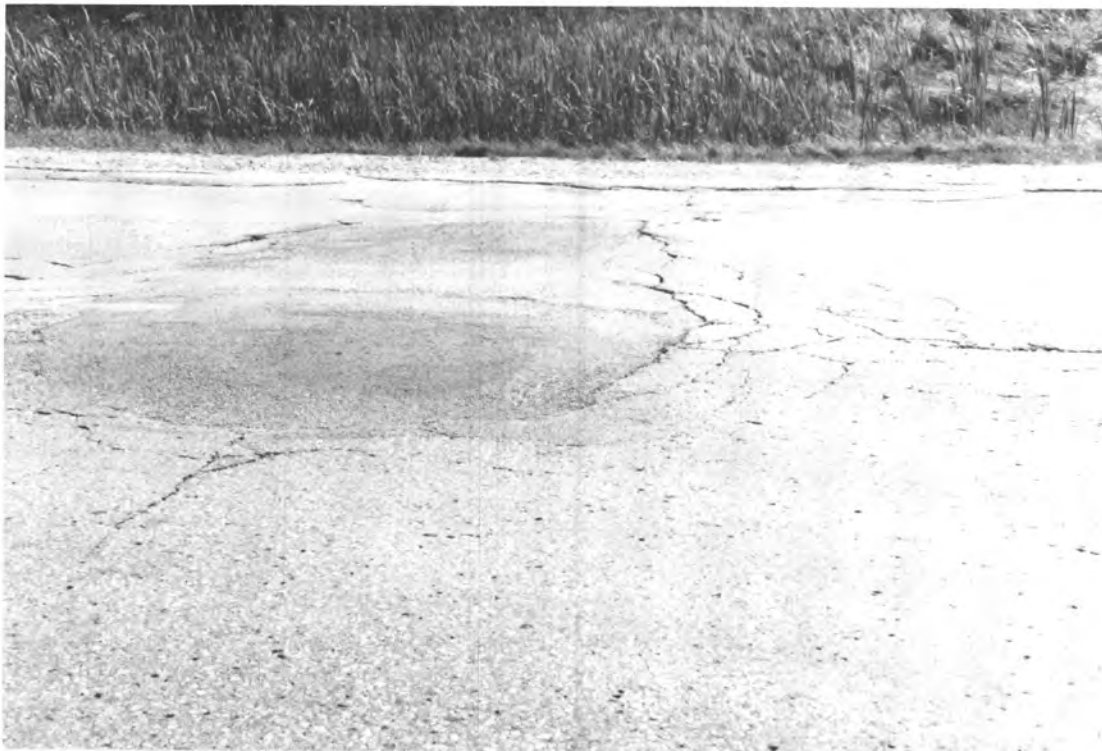
Severe Distortion from Frost Heaving
