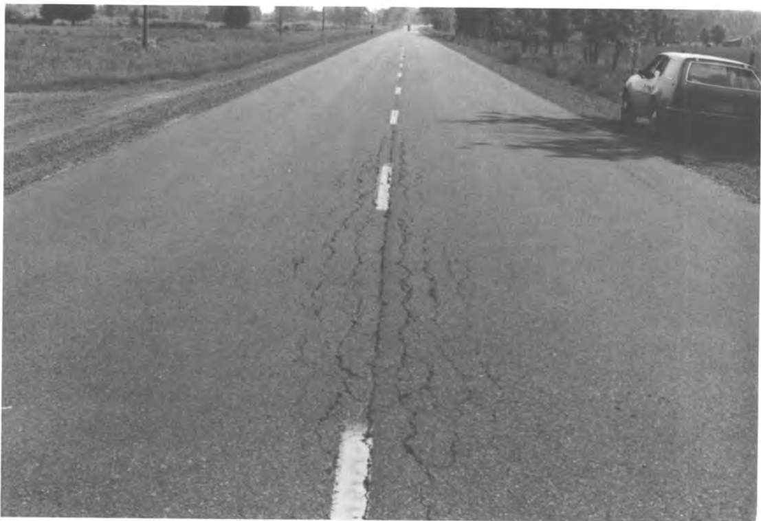
Moderate (Multiple) Centre Line Crack
