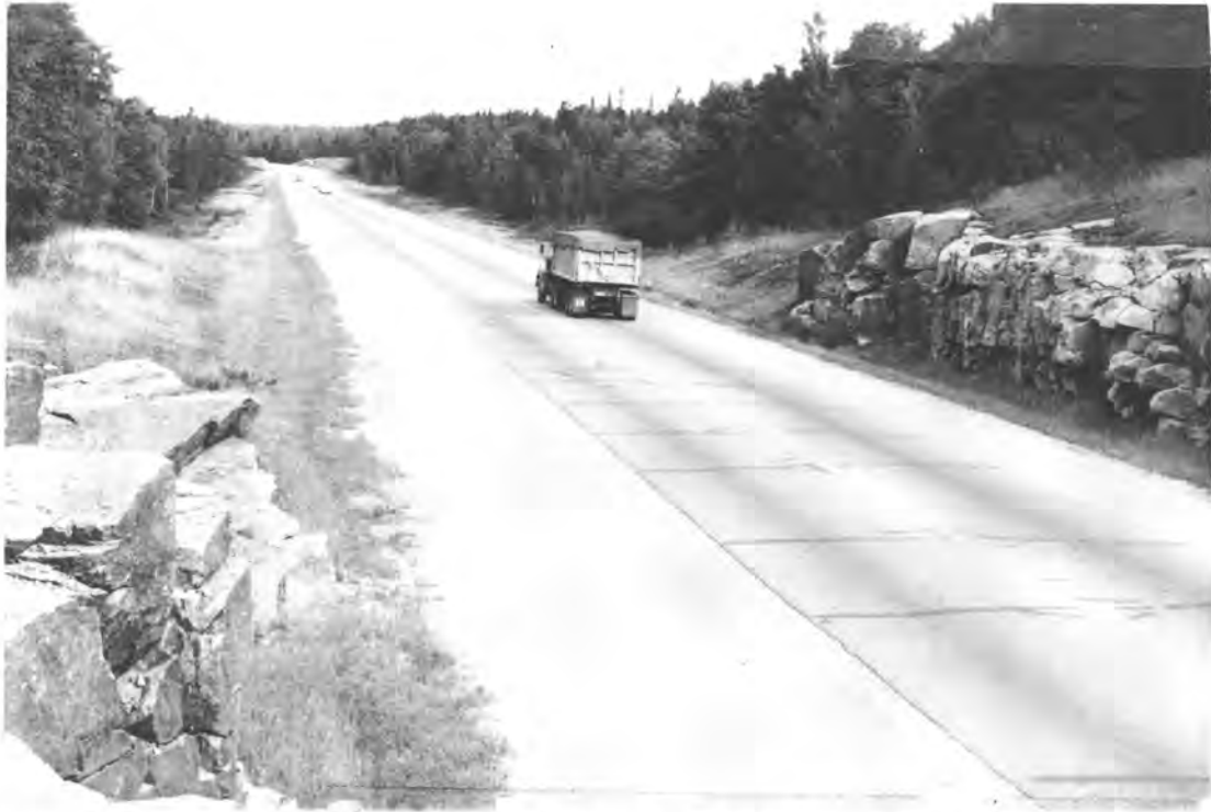
Typical Transverse Crack Regularly Spaced along the Length of the Roadway
