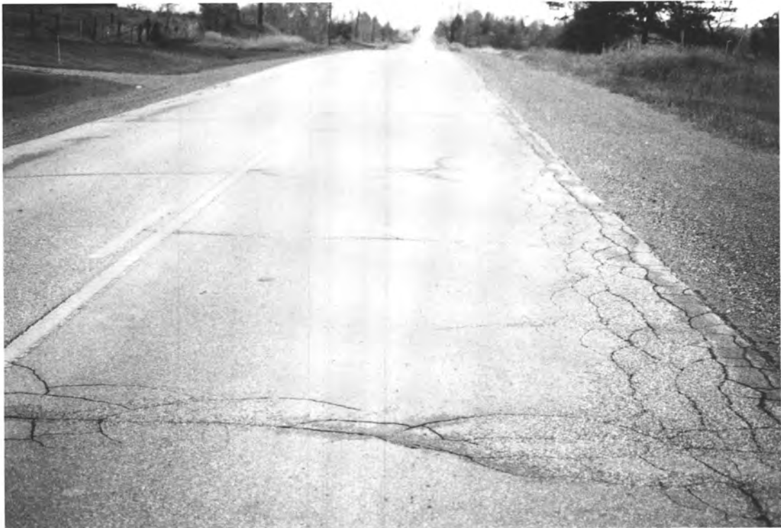
Riding Condition Rating: Poor
