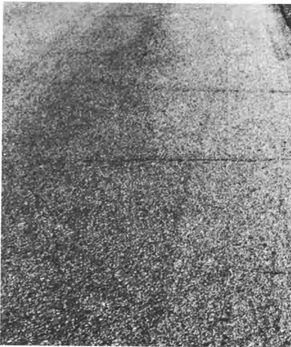
Very Slight Partial Transverse Crack
