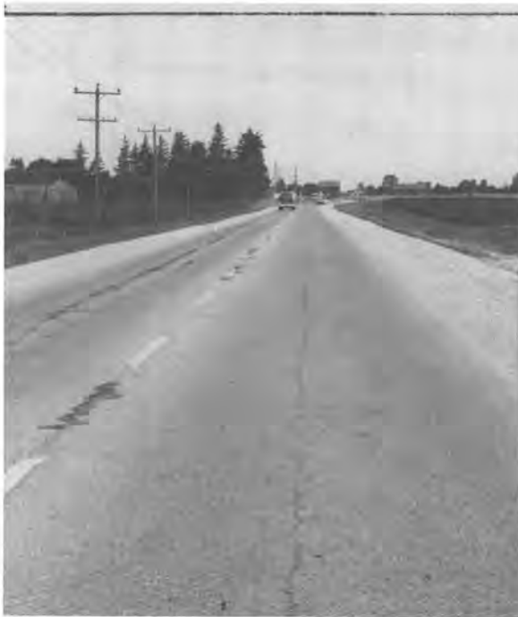
Slight Longitudinal Mid-lane Crack
