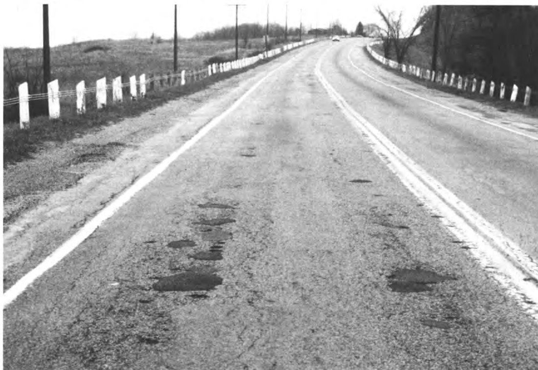
Riding Condition Rating: Very Poor
