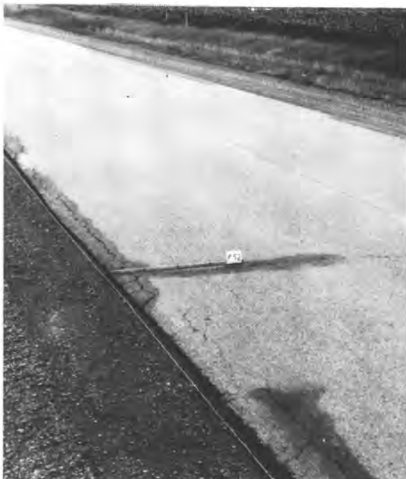
Very Slight Pavement Edge Crack
