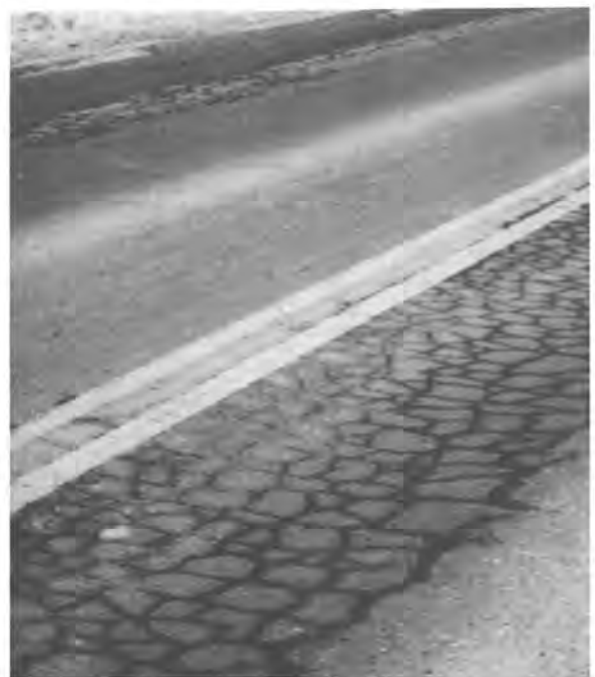
Slight Alligator Crack (Wheel Track Longitudinal Crack)
