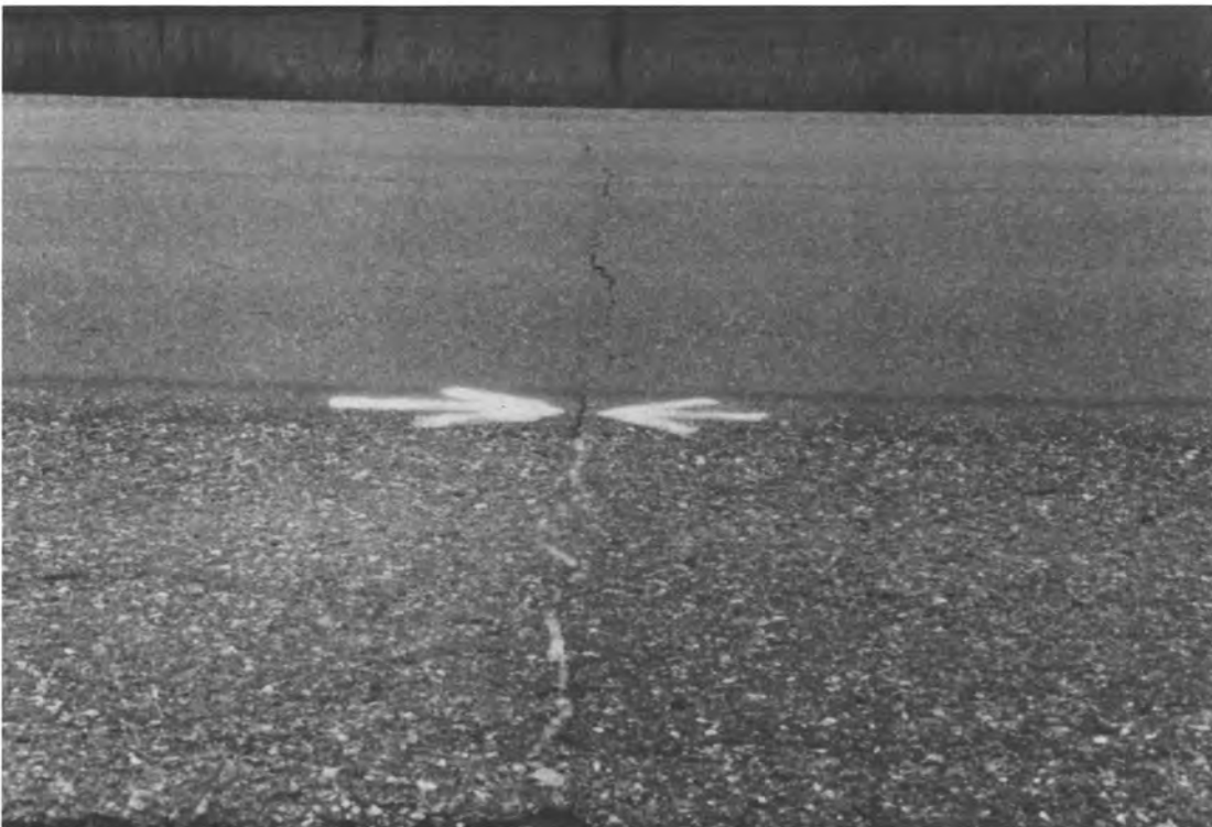
Transverse Crack of Surface Treated Shoulder
