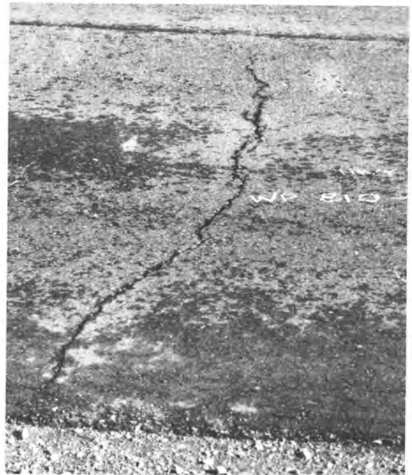
Slight Half Transverse Crack
