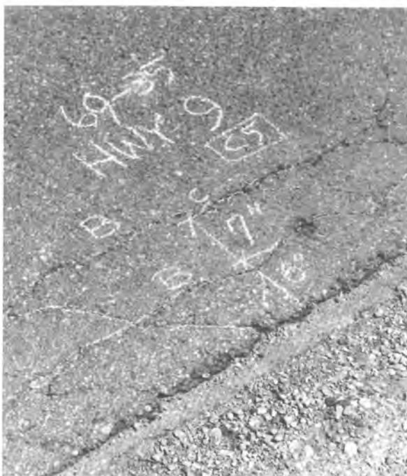
Moderate (Multiple) Pavement Edge Crack
