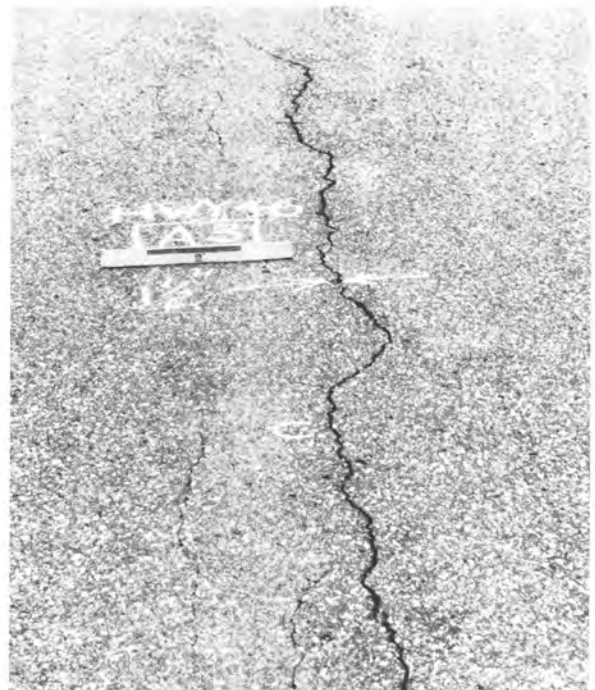
Moderate (Multiple) Longitudinal Mid-lane Crack
