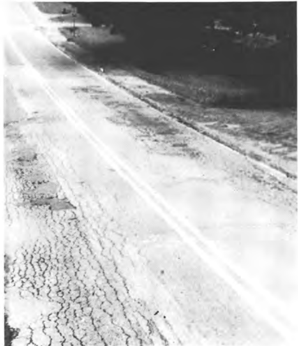
Very Severe Pavement Edge Crack
