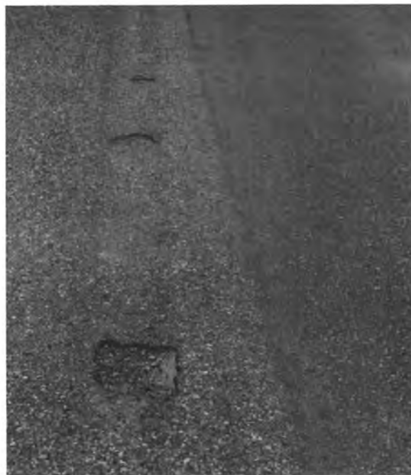
Breakup of Stabilized Shoulder
