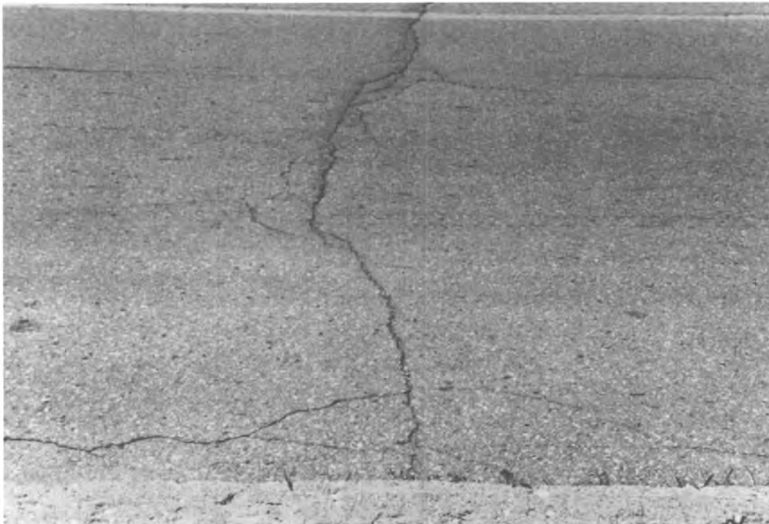
Moderate (Multiple) Transverse Crack
