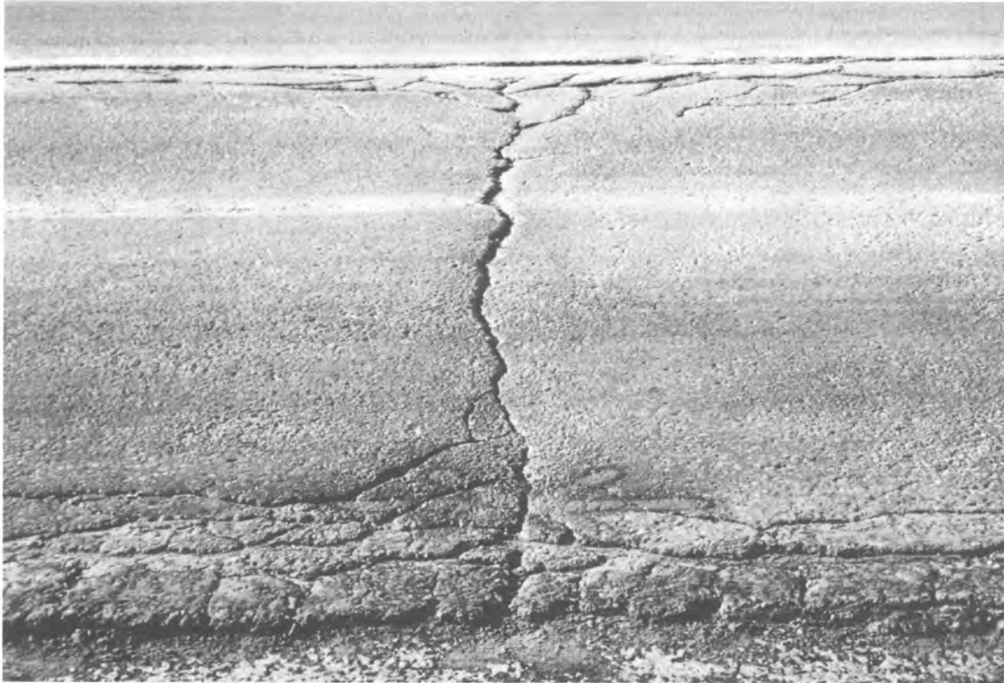
Severe Distortion from Transverse Crack Cupping
