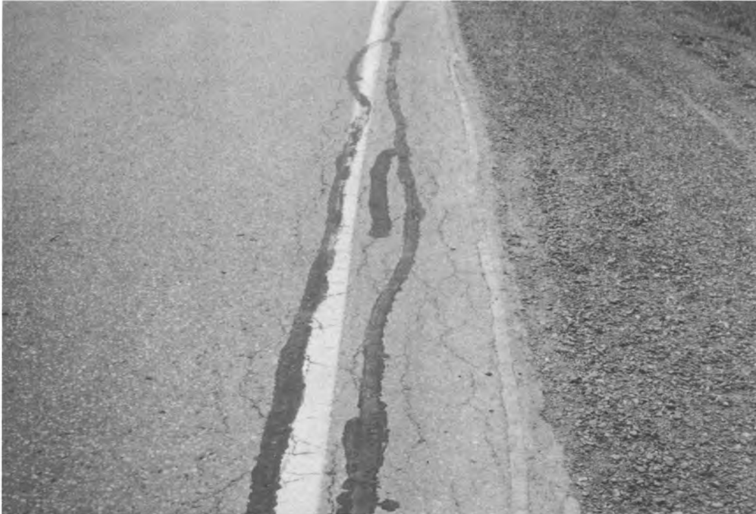
Paved Shoulder Cracking
