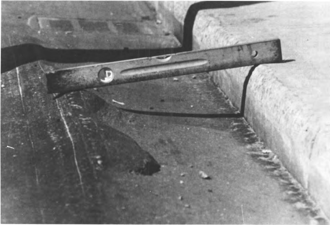
Very Severe Shoving
