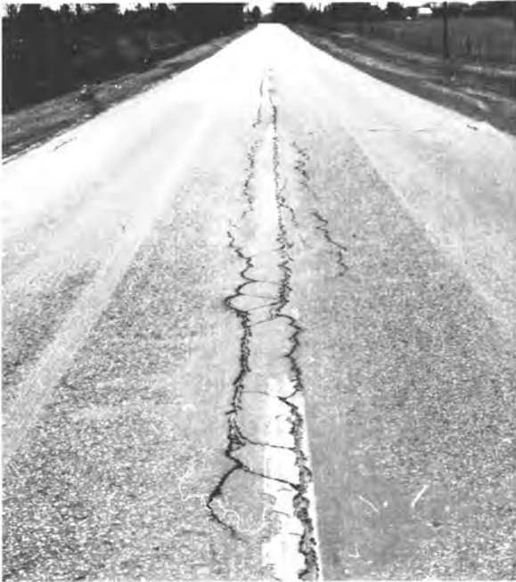
Severe (Multiple) Centre Line Crack
