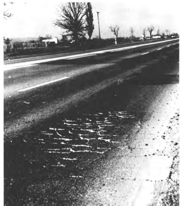
Very Severe Alligator Crack *
