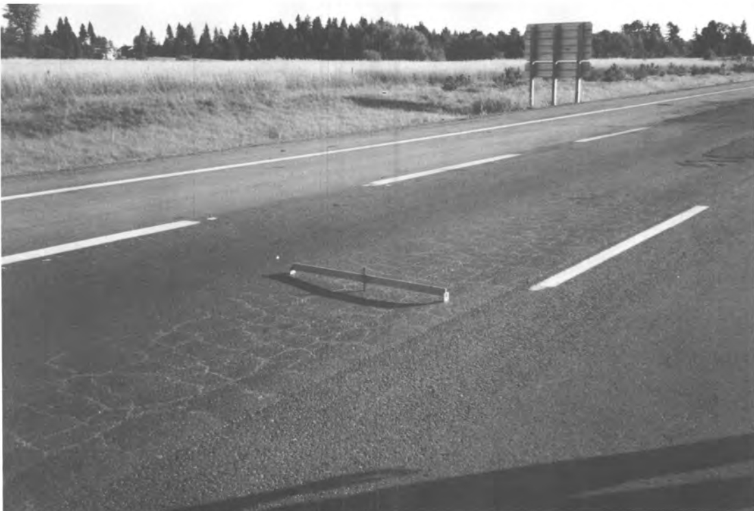
Very Severe Distortion from Subgrade Failure
